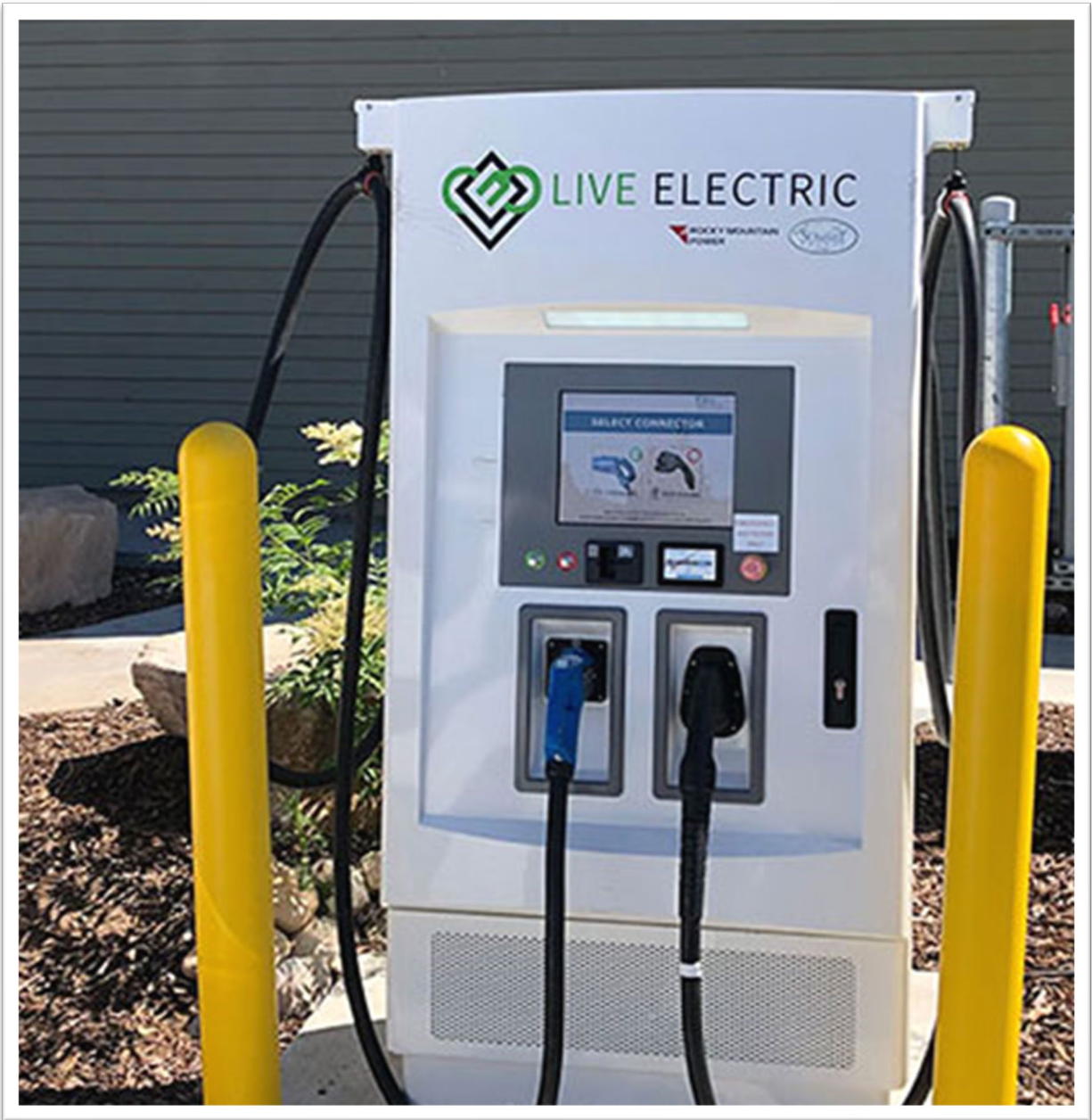
Photo courtesy US DOE Alternative Fuels Data Center .
